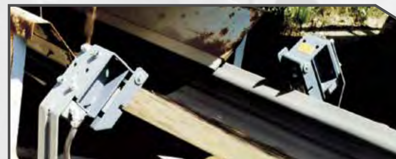
Shown are two BA units protecting a valuable conveyor belt from damage due to belt misalignment or run-off at an aggregate facility
