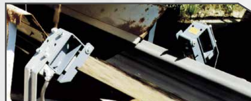
Shown are two BA units protecting a valuable conveyor belt from damage due to belt misalignment or run-off at an aggregate facility
